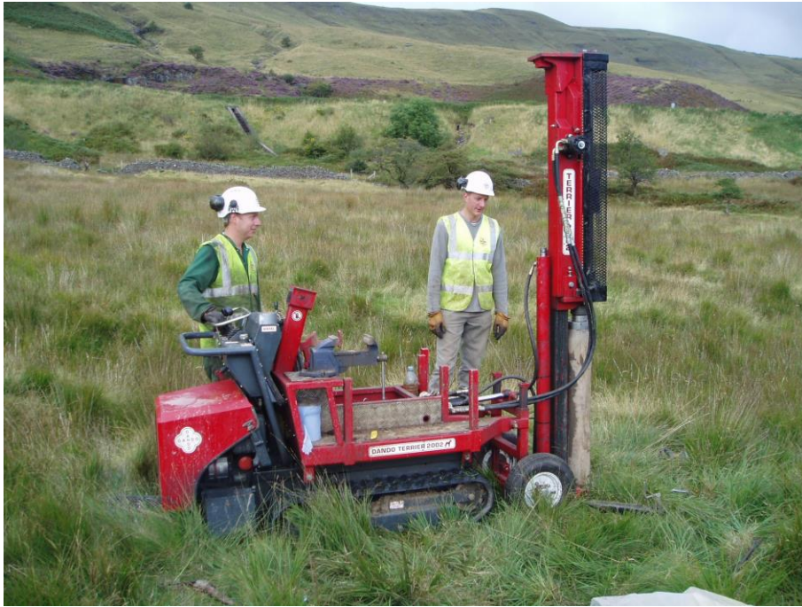
BGS Dando drilling rig drilling two boreholes to bedrock through the peat filled basin
