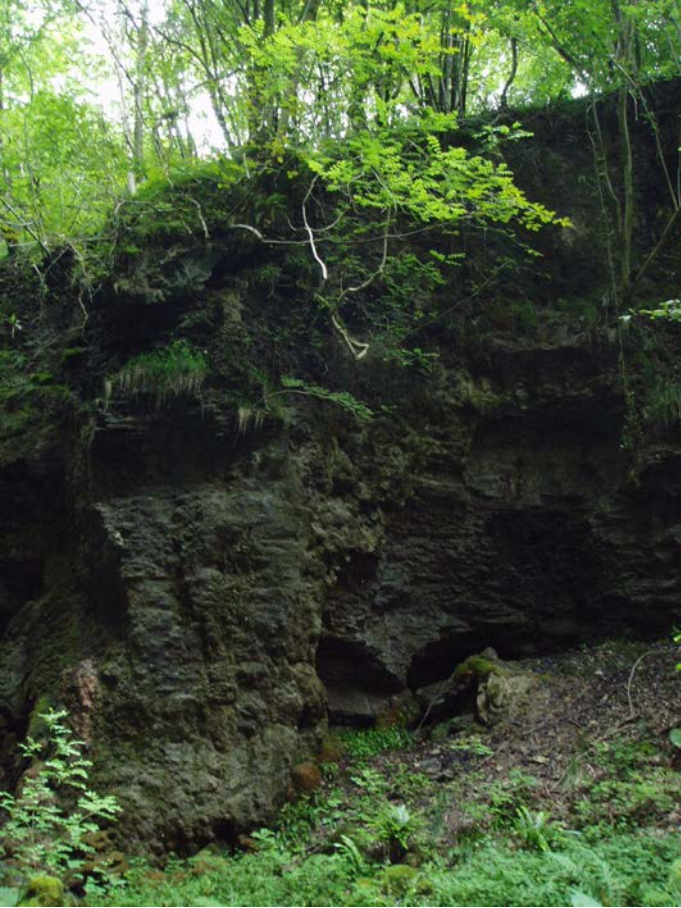
The sides of the Nant Ffrwd gorge are vertical, with loose overhanging sections
