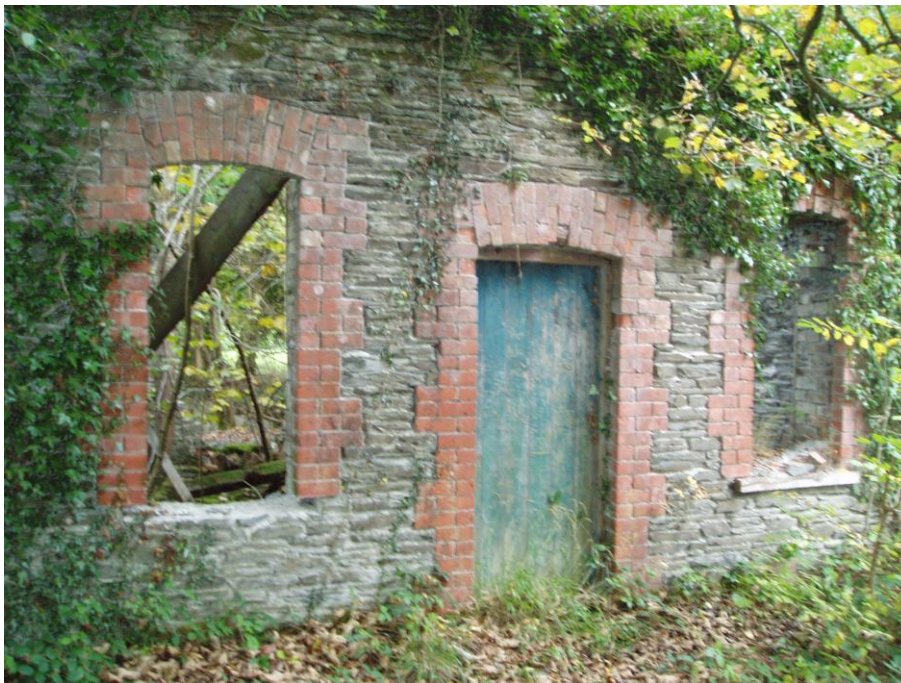
West facade of Barium Well pump room facing onto a small terrace
