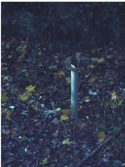
Standpipe in floor of Barium Well wellhouse
