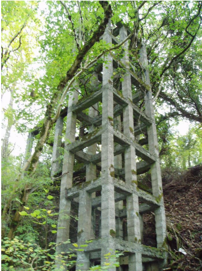
Curious early 20 th century concrete structure – possible a water tower or an uncompleted elevator which was intended to lead to the Chalybeate Spring from the lane above.
