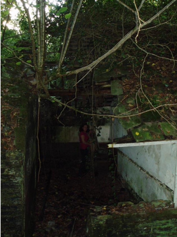
The pump room – note collapsed roof
