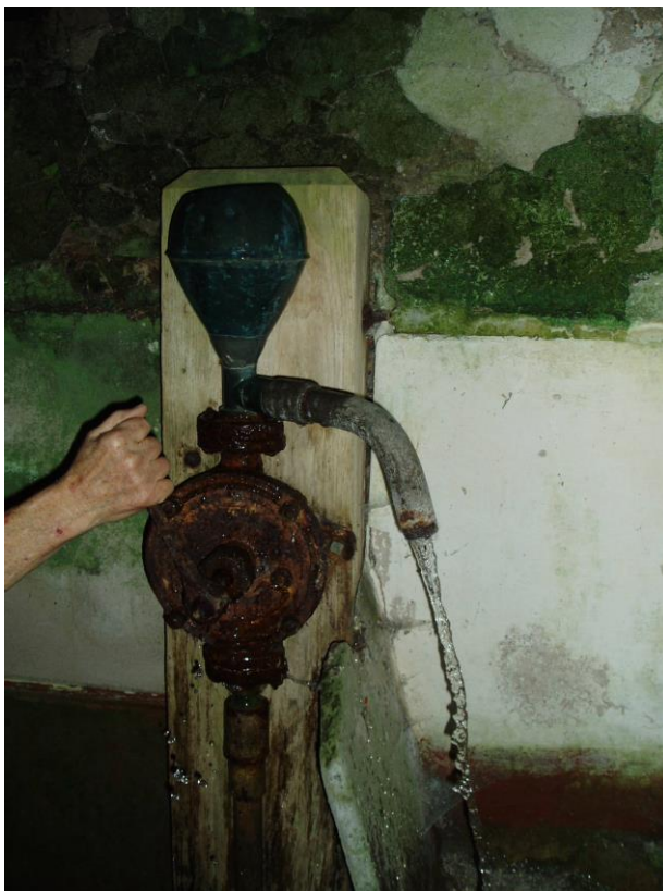
The flowing pump
