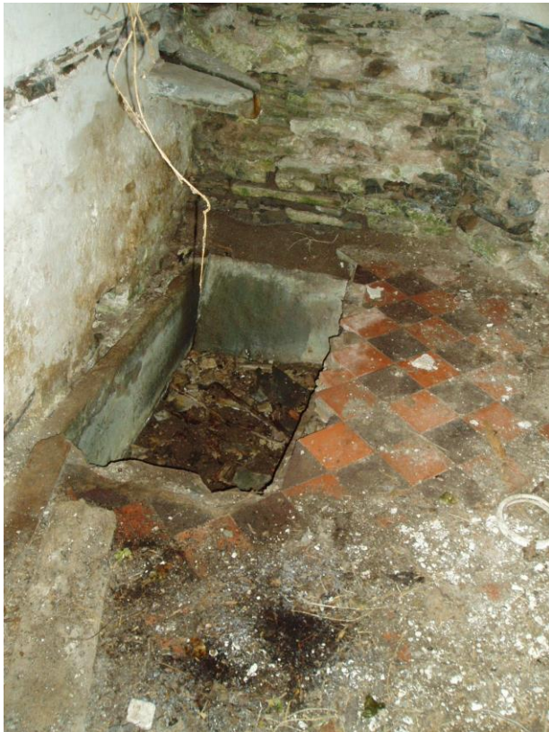
The bath with the water inlet above from the pump room next door
