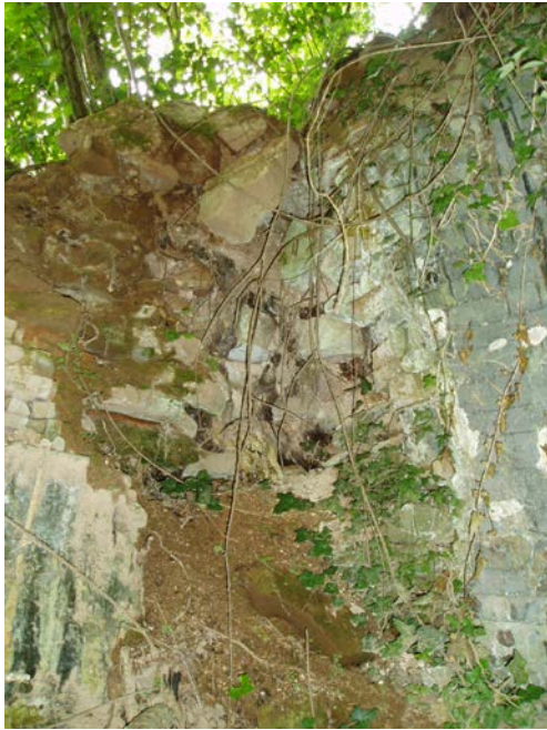
Charging hole which has collapsed since 1970's
