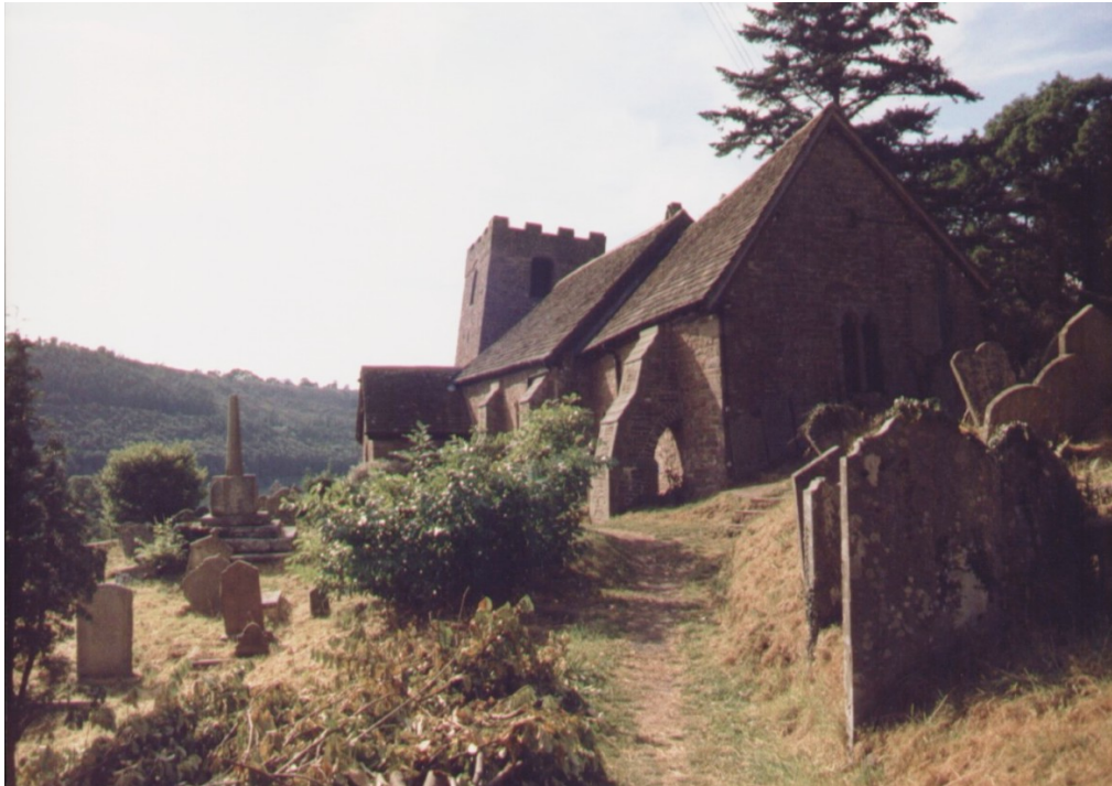
View showing the distortion of Cwmyoy village church caused by ongoing movement of the Cwmyoy landslide. Note buttresses supporting the walls. As each part of the church was built, attempts were made to counter previous movements, resulting in a building with different parts at different angles. Photograph: A. Humpage
