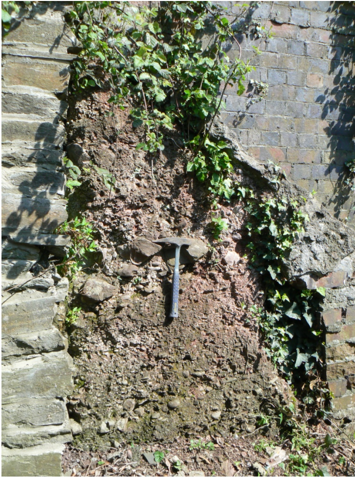
The Llanishen Conglomerate as it appears in a retaining wall on the Eastern side of the railway line behind the waiting shelter
