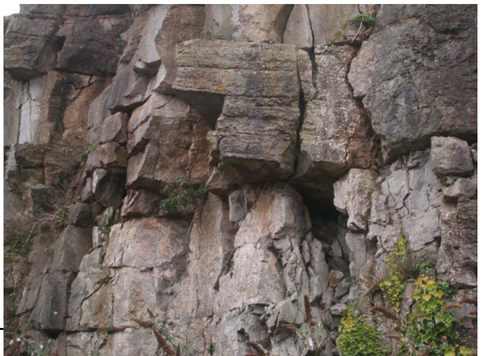
Photograph 4. Close up of the base of the overhanging base
